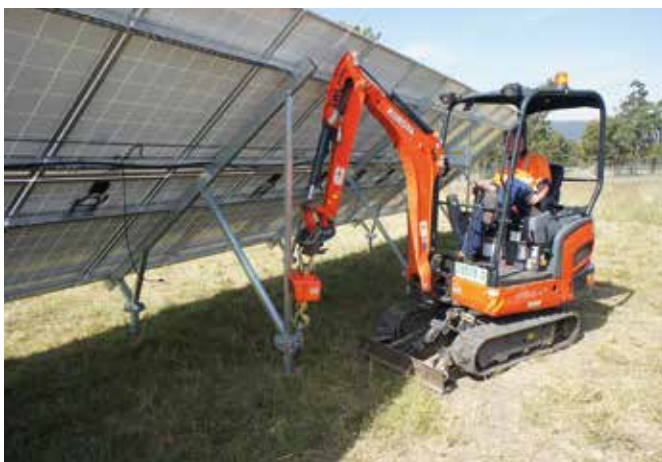
Installation des Solarsystems am Sendemast in Muswellbrook – Installation of the solar power system at the transmission mast in Muswellbrook
